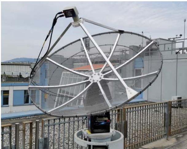
Rotating satellite dish on the roof of the Geodesy Building used to analyse the signal patterns of signals of opportunity © IFG/TU Graz
